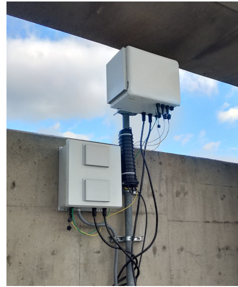
Figure 7: 160-radio weatherproof ArgosV3 base station deployed at Rice University stadium.
